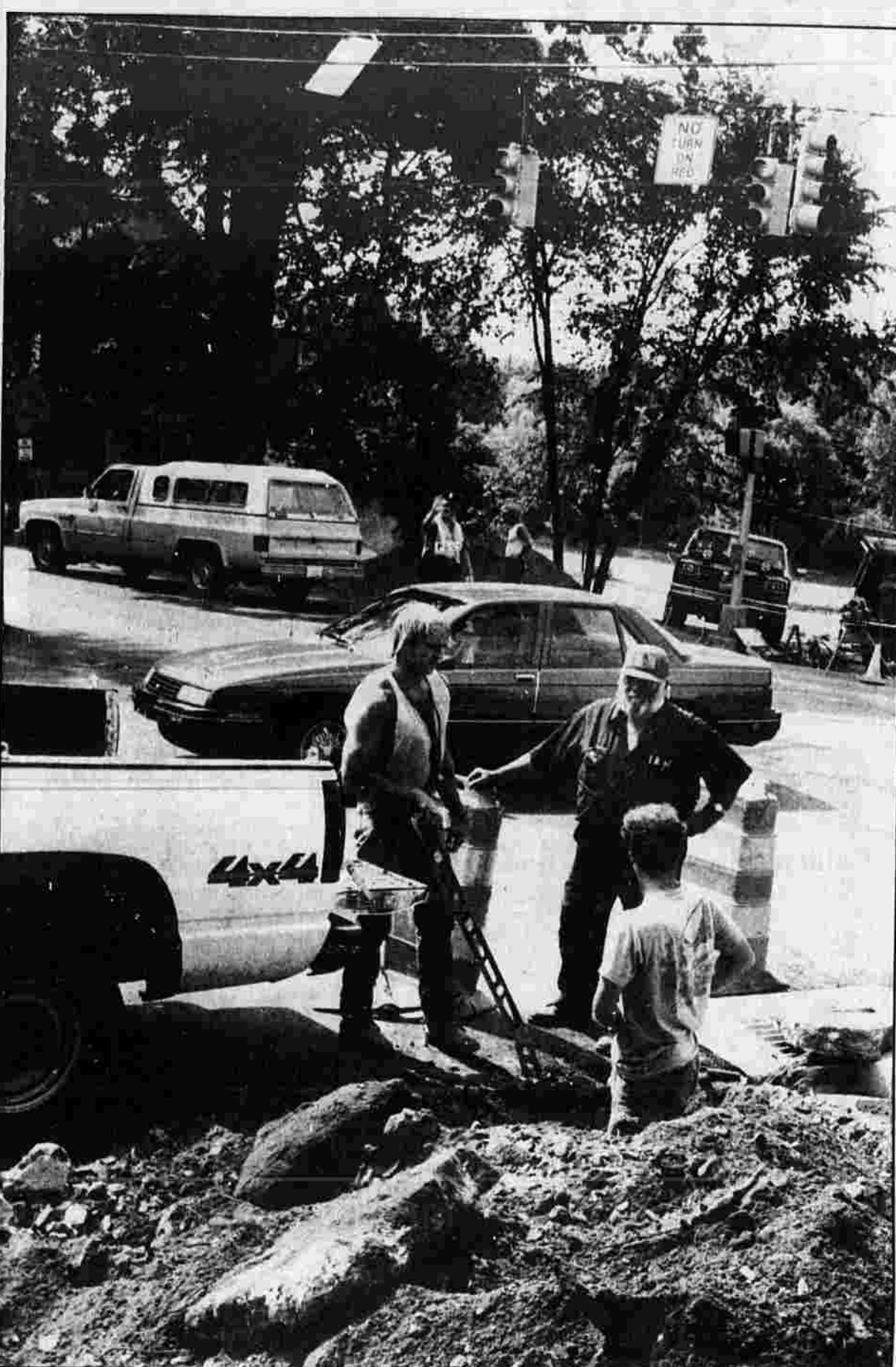
TOUGH WORK —Bob Wassik of Plainville, Richard Blacenza of Springfield, Mass., and Jeff Hazard of Simsbury are installing electrical wiring at the corner of Spruce Street.
